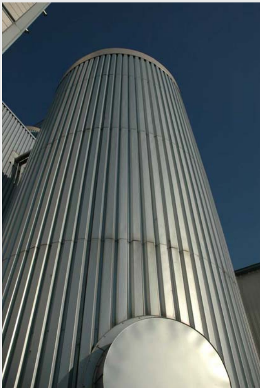
CO 2 Cuve de stockage 90 to
