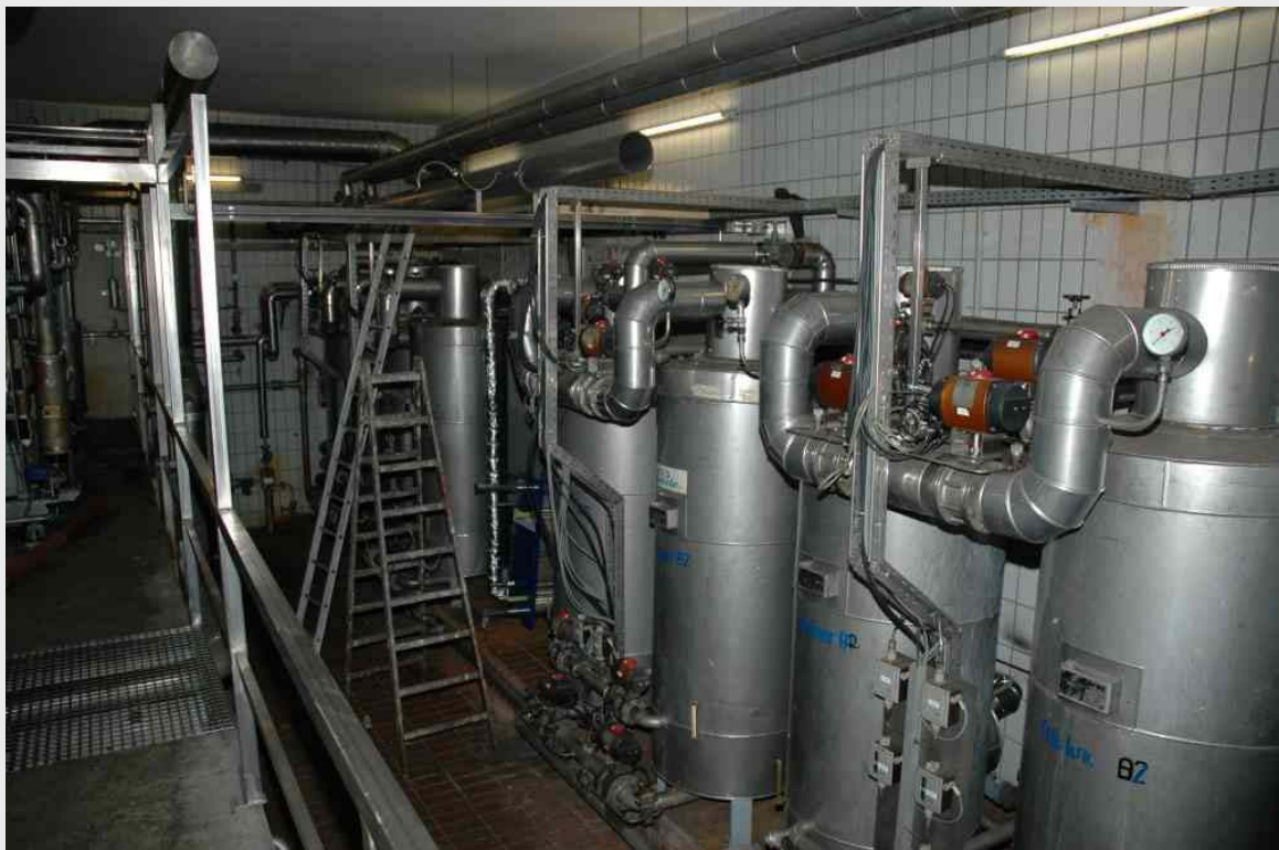
CO 2 Dryer and Cleaner
