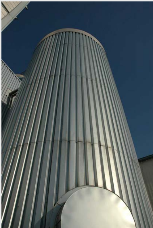
CO 2 Lagertank 90 to
