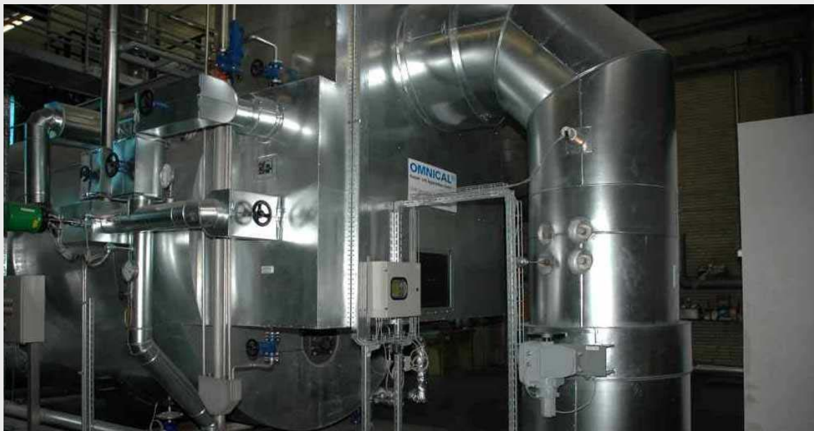
Steam Generator 18 toph
