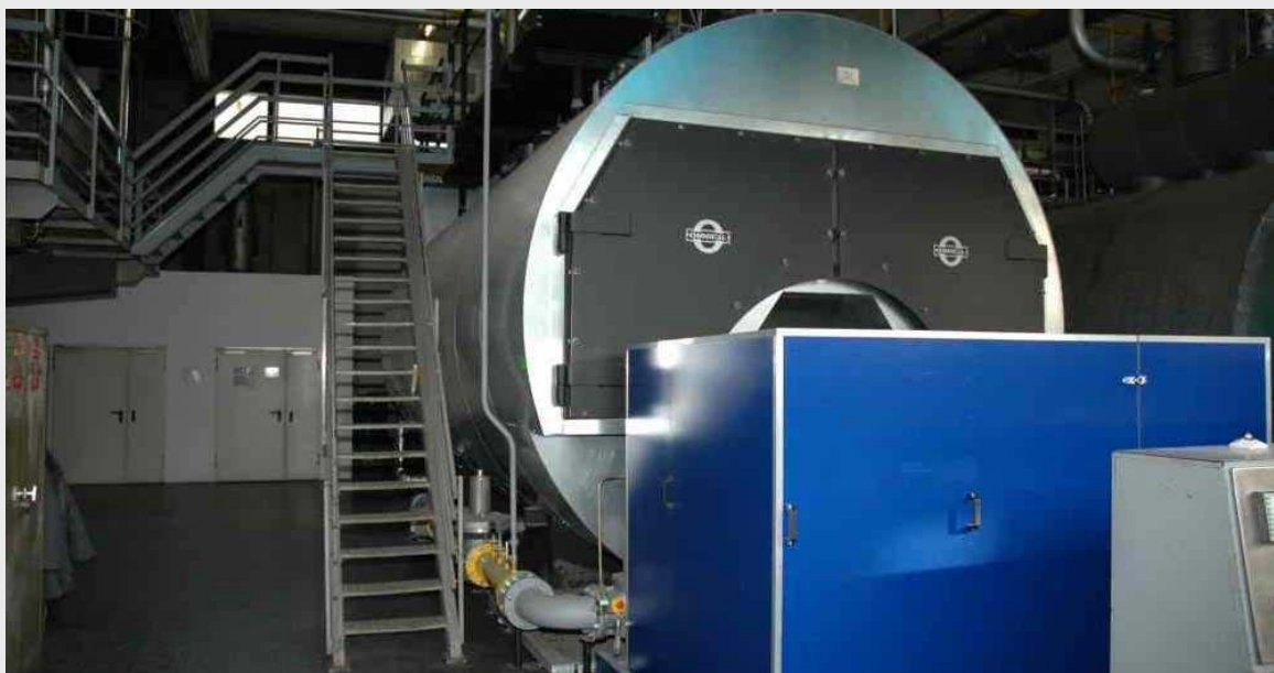
Steam Generator 18 toph
