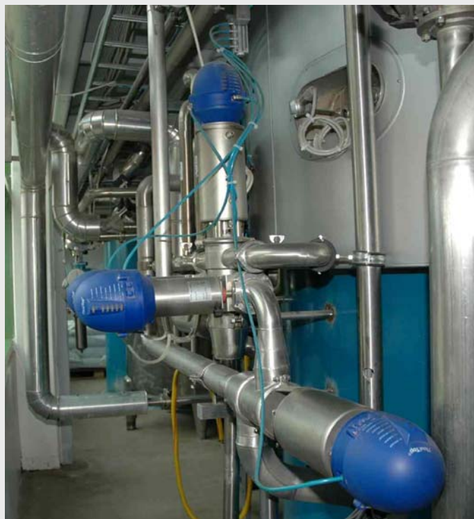
Brewhouse – Diverse Valves
